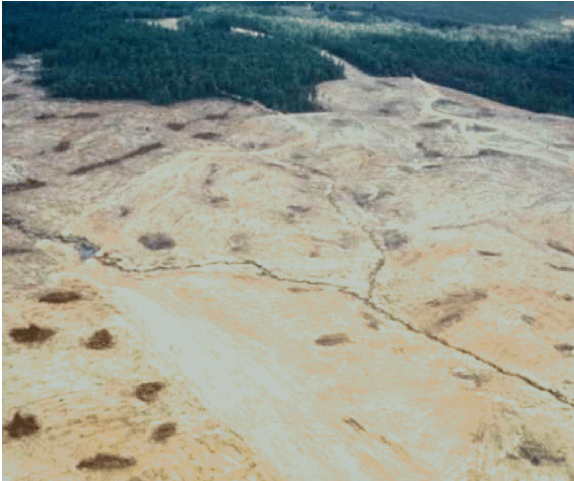
The clearing of Lake Anna's bed started in 1968. This photo captures the clearing of the lake bed where the Pamunkey Creek and North Anna River intersect at Spotsylvania and Louisa County.
